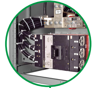
Fig. 13: Ground and neutral disconnect links
